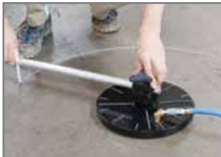
Set up vacuum base and mark cut with soap stone by rotating pivot bar
