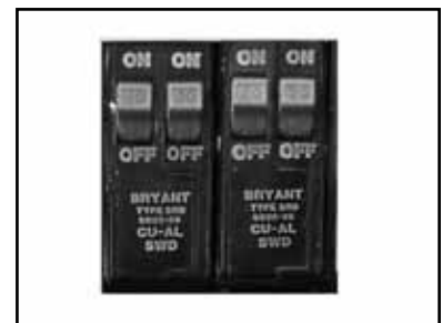
(C) Verify circuit breaker is not tripped, if it is tripped – reset the circuit breaker once.
